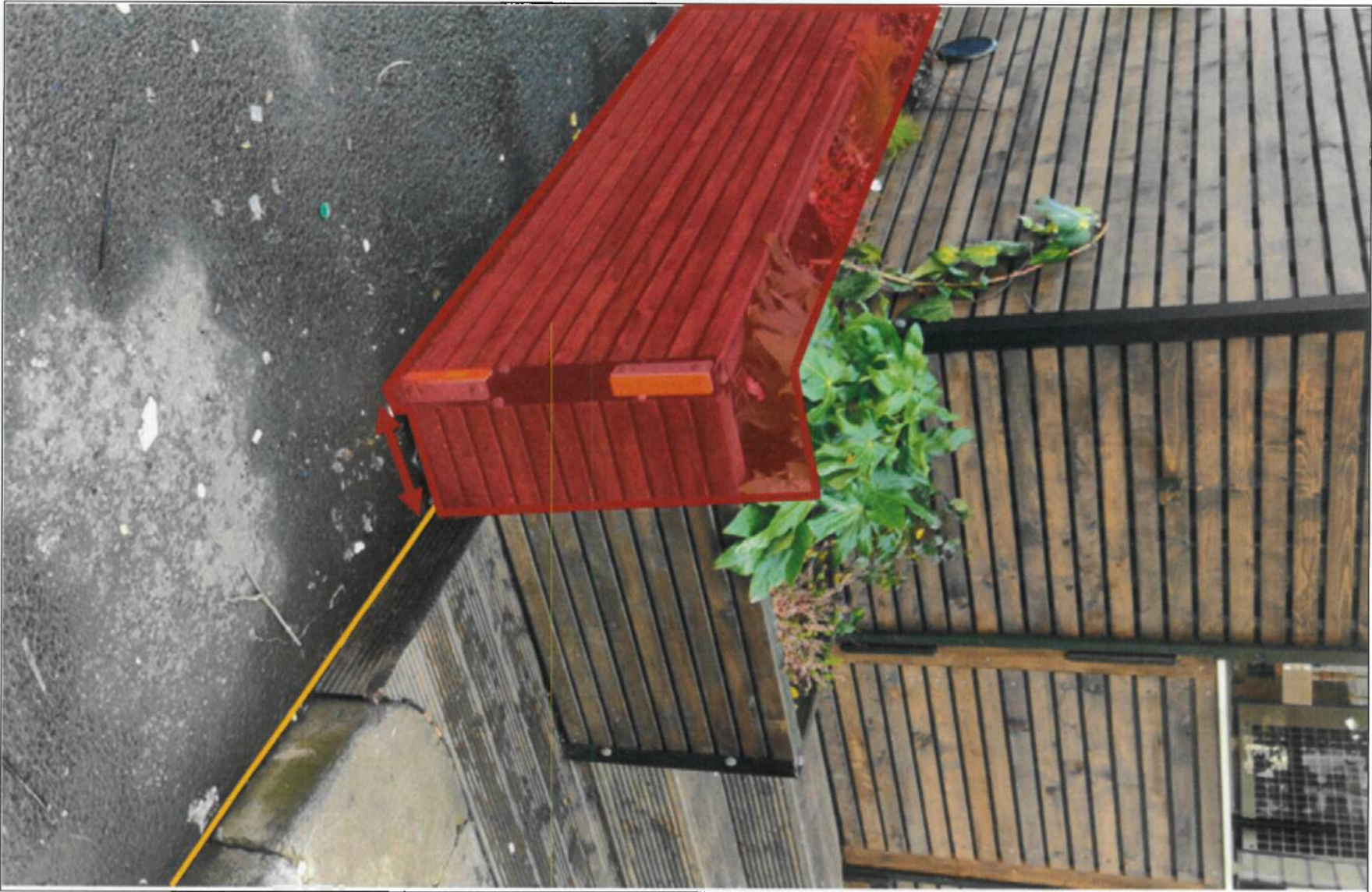
Figure 5.3: Picture showing the protrusion of the café approximately 30cm outside the footprint of the suspended Loading Bays. (Source: Tom Phillips + Associates, January 2023.)
