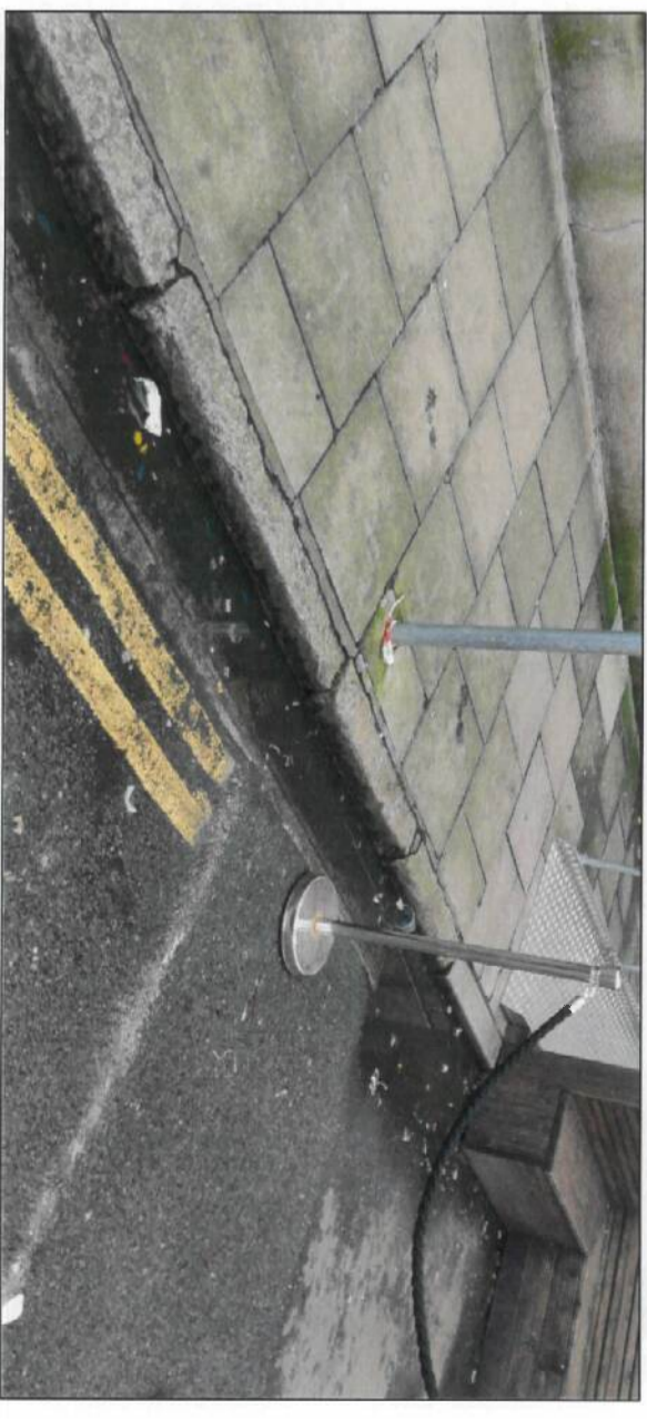
Figure 5.5: Standing water on Clonmel Street as a result of having the on-street stormwater drain being covered by the RSC. (Source: Tom Phillips + Associates, January 2023.)
